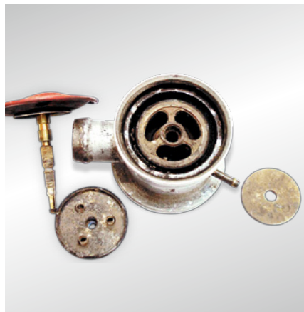
Fig. 30: cut-off secondary air valve – damage to the diaphragm and valve plate due to condensates
