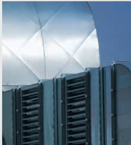
Installation de ventilation
