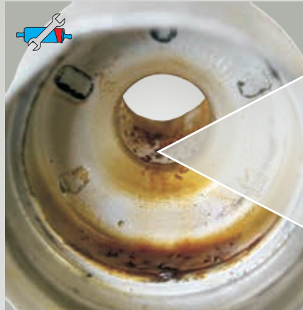
Fig. 64: Crystalline deposits caused by unsuitable fluids
